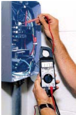
Testing for Voltage...anything wrong with this picture?
